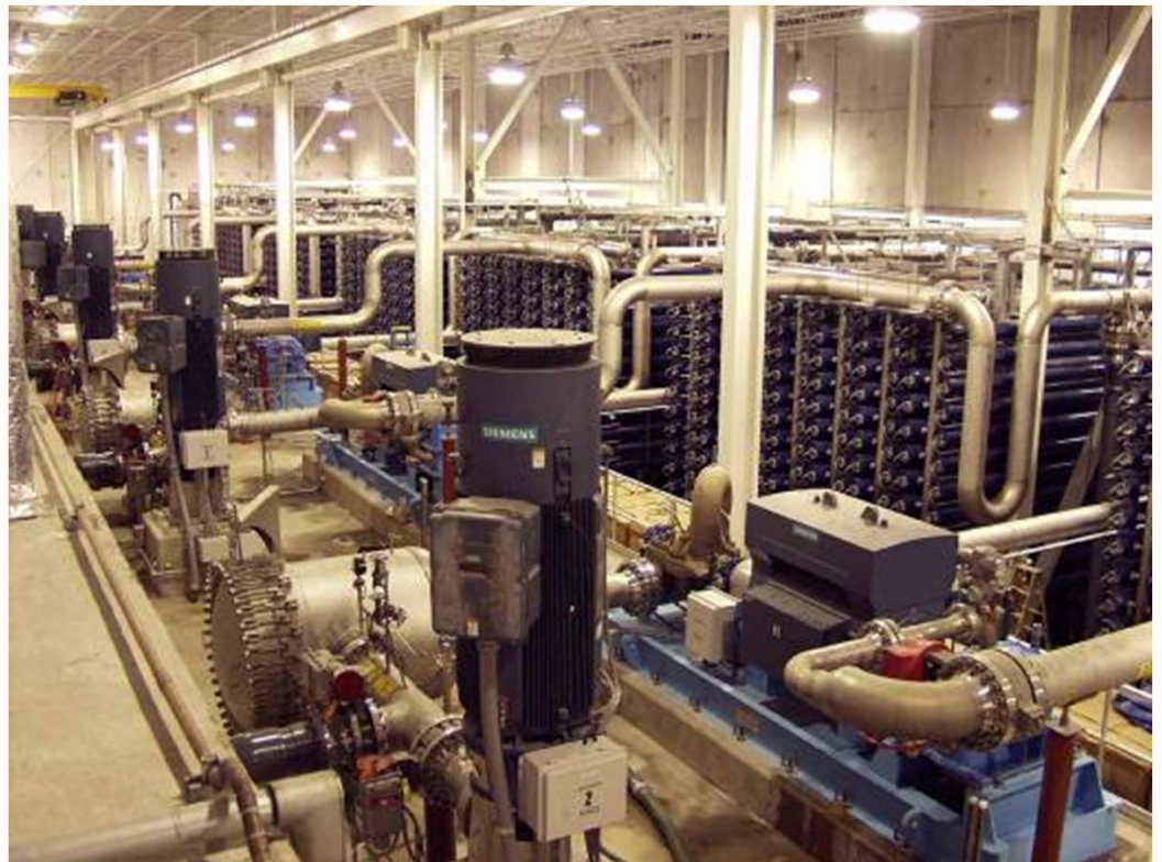
Tampa Bay Water Desalinization Facility
